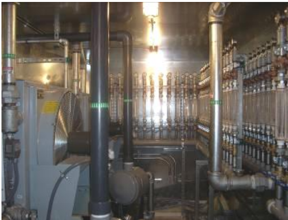
SVE/Air Sparge System
