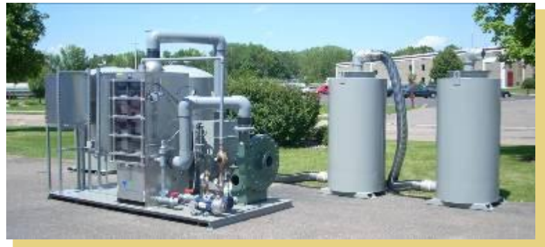
Low Profile Air Stripper Skid w/ VGAC off gas Treatment
