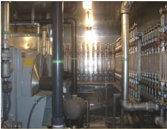
SVE/Air Sparge System
